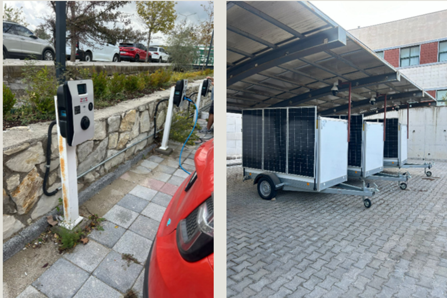
Figure 6. EV battery chargers and mobile chargers from left to right
