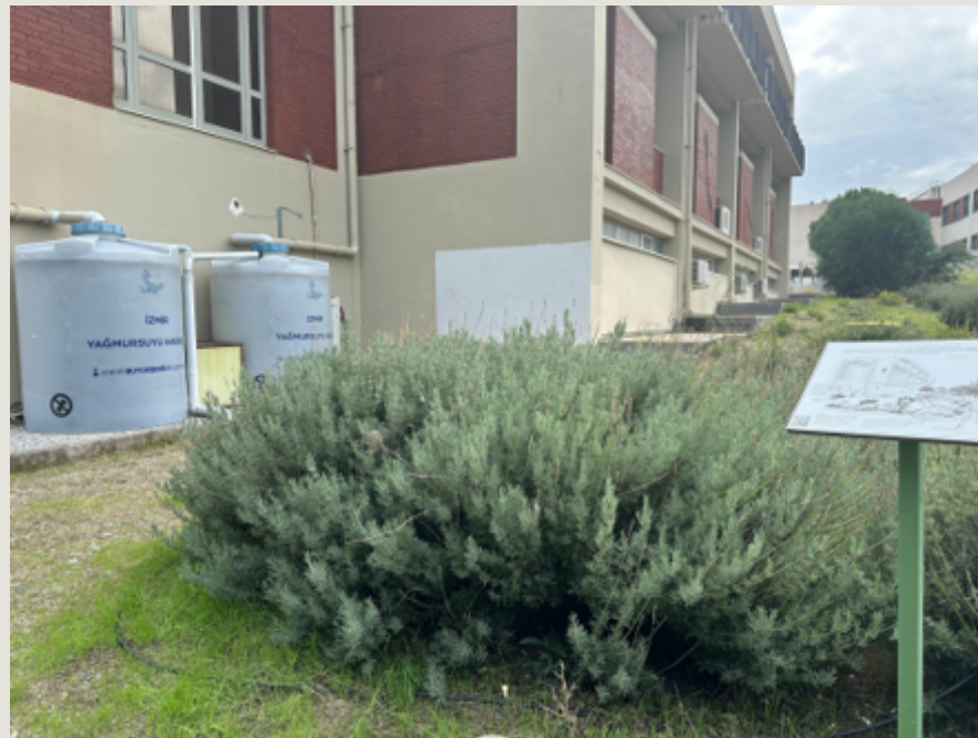
Figure 4. Rainwater Harvesting Tanks
